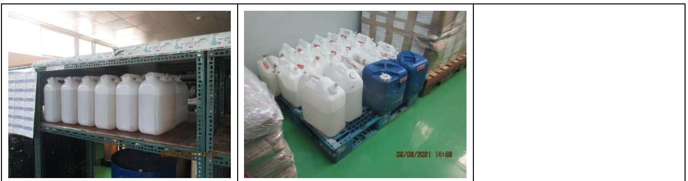
NC: Some chemicals (oil) were not adequately stored with 2nd container. NC: Some chemicals (oil) were not adequately stored with 2nd container.
